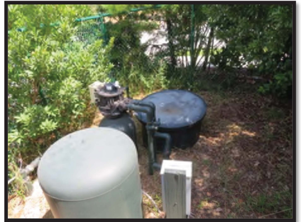
Figure 5 30A Landscape and Lighting
